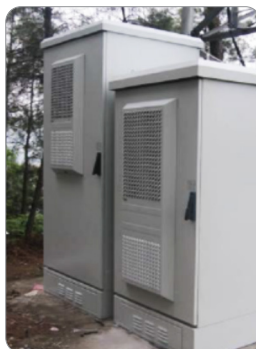
2. Mobile base station communication cabinet
