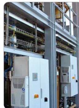
4. Power switch cabinet
