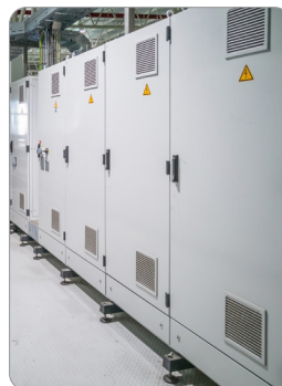
3. Electric control cabinet of industrial factory
